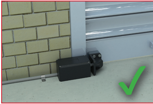
Lock mounted to the ground.
